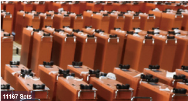
Location: South Africa Time: 2025 Application: Telecom Project
