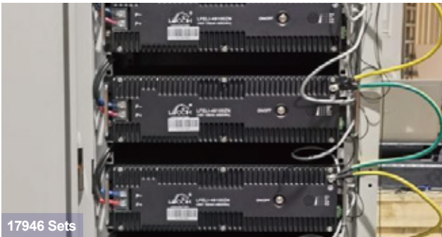
Location: Australia Time: 2022 Application: Telecom Project
