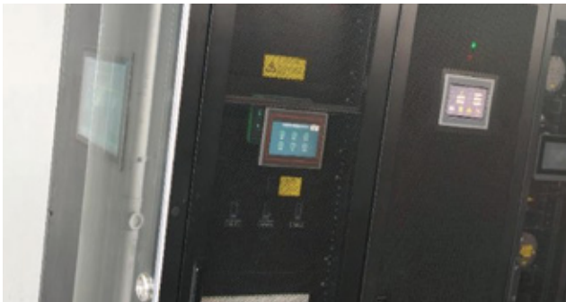
Location: China Time: 2024 Application: Tsingtao Brewery Data Center
