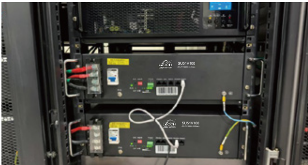
Location: China Time: 2025 Application: AITWELL UPS
