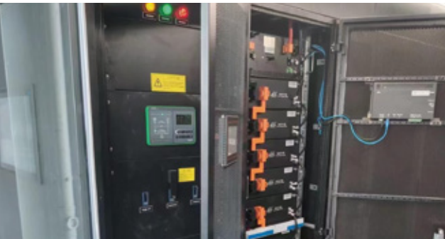
Location: Hong Kong, China Time: 2024 Application: Data Room Supporting
