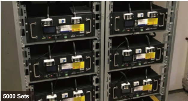
Location: United Kingdom Time: 2019 Application: Telecom Project
