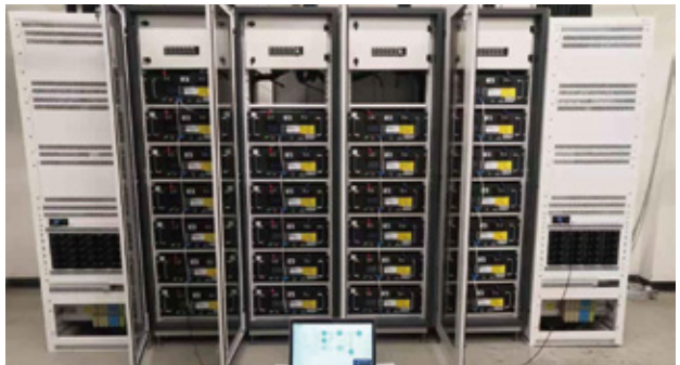
Location: Thailand Time: 2023 Application: Data Room
