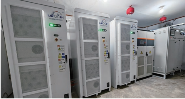
Location: Sulawesi, Indonesia Time: 2025.1 Application: Remote Island Off-Grid Microgrid
