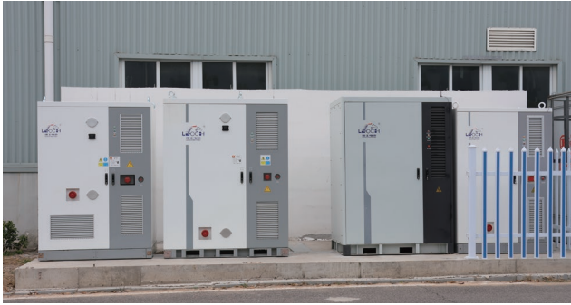
Location: China Time: 2024.8 Application: Peak Shaving and Valley Filling
