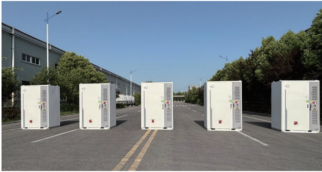
Location: China Time: 2025.7 Application: Peak Shaving and Valley Filling
