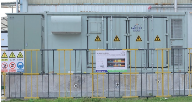
Location: China Time: 2026 Application: Peak Shaving and Valley Filling
