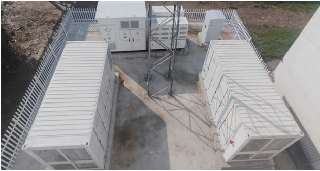
Location: China Time: 2024 Application: Peak Shaving and Valley Filling
