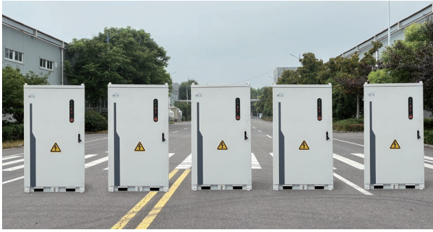
Location: Germany Time: 2025.9 Application: Photovoltaic Energy Storage
