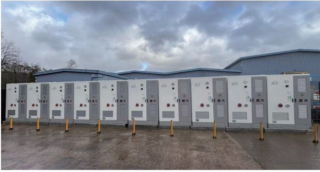
Location: UK Time: 2025.12 Application: Distributed Energy Storage
