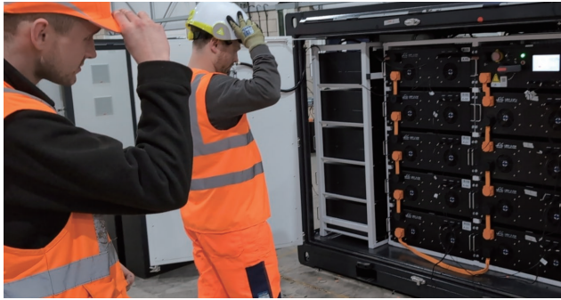
Location: China Time: 2025 Application: Peak Shaving and Valley Filling
