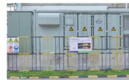
Location: China Time: 2026 Peak Shaving and Valley Filling 2.089MWh
