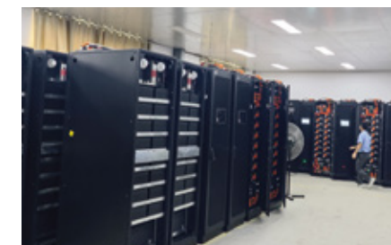
Location: China Time: 2025 Data Room RU6-512V200
