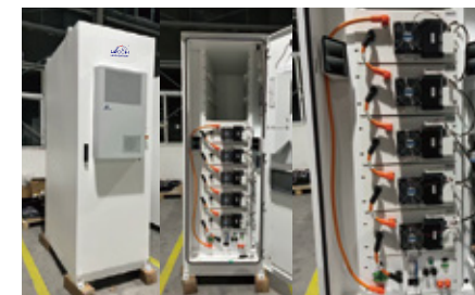
Location: Dominican Time: 2026.03 Dominican Energy Storage 1300kWh
