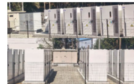
Location: Japan Time: 2025.5 Peak Shaving and Valley Filling 16.68MWh
