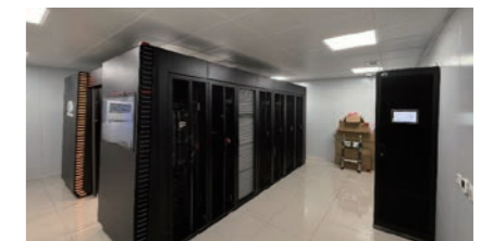
Data Room Project Location: Inner Mongolia, China Solution: PU512V160Ah 2 Sets
