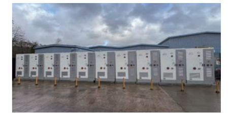
Distributed Energy Storage Project Solution: United Kingdom Solution: 105KW/232KWh 10 Sets
