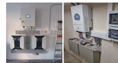
Home Storage Project Location: South Africa Solution: LFELI-48100TB/LFELI-48100S/ LFELI-48100S2 8200 Sets
