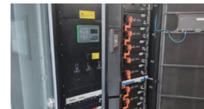
Data Room Supporting Project Location: Hong Kong, China Solution: PU512V100Ah 20 Sets
