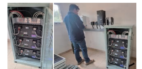
Renewable energy projects Location: Argentina Solution: LR51.2-100/LR51.2-200/ LR25.6-200+Battery cabinet 425 Sets
