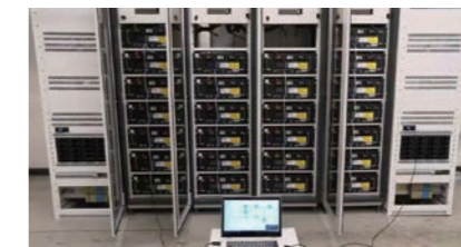
Thailand Data Room Location: Thailand Solution: SU192V25 13 Group
