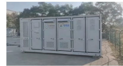
Electric Vehicle Charging Project Location: Hong Kong, China Solution: 300KW/645KWh 10 Sets
